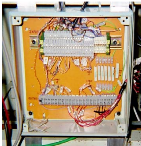
Fig. 5-4: Sets of Electrical Connectors for the VBF System (AMTLAB)
