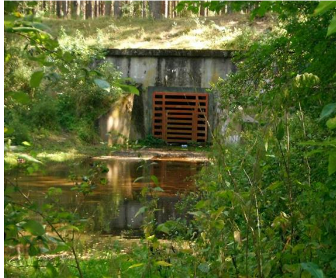
Figure 3.31 Evidence of flooding at the entrance to section 6 during the September 2013 survey.
