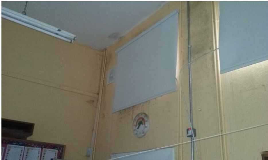
Figure 7.10 Evidence of mould growth on the north-facing wall of Classroom3.
